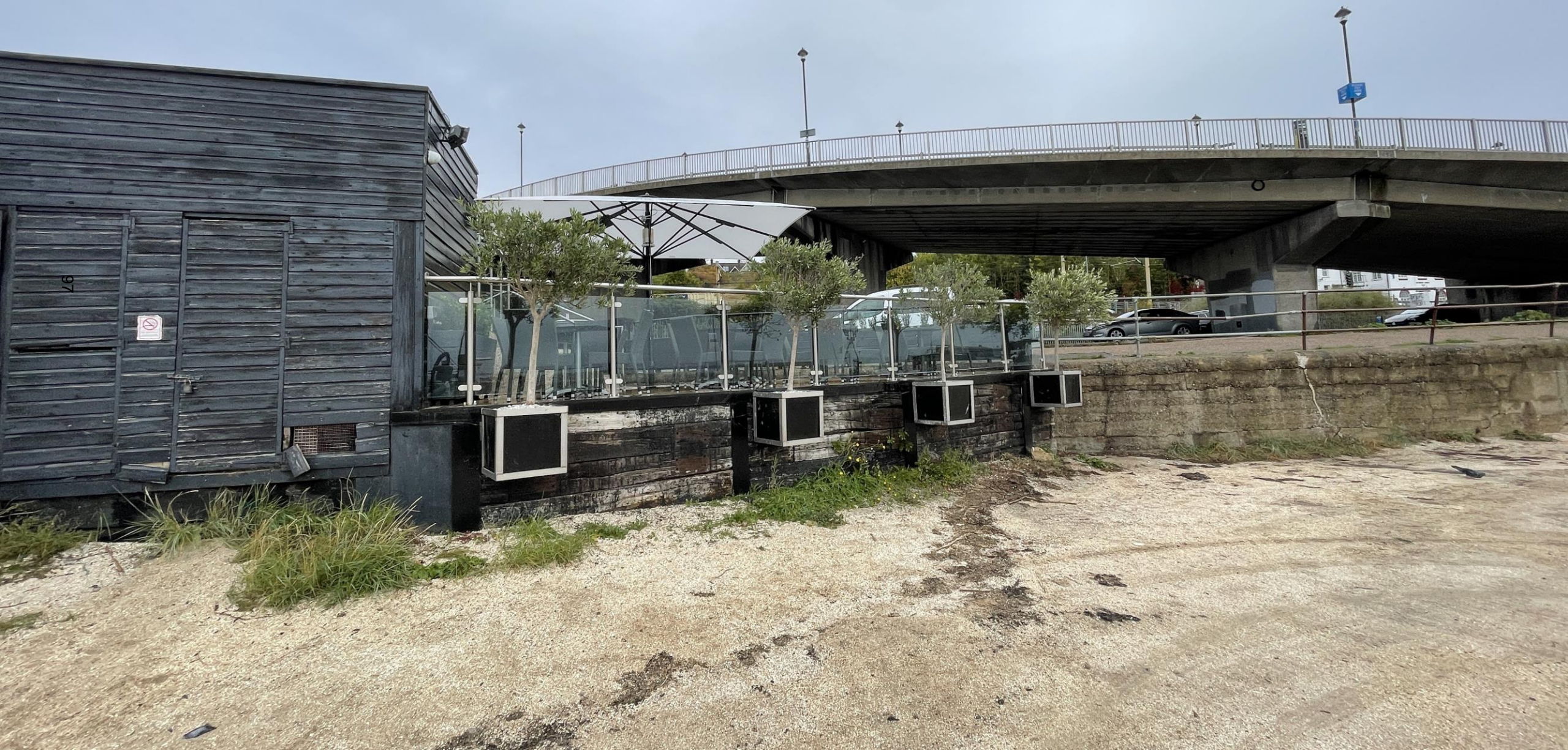
South Elevation showing Existing External Terrace and Existing Doors to Storage Area
